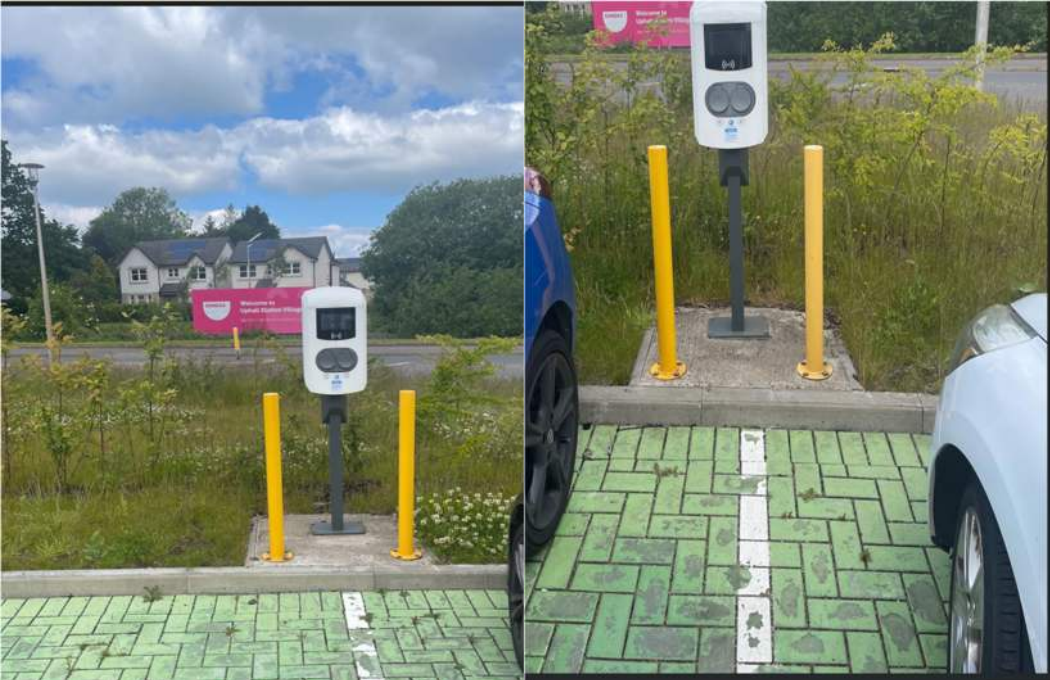
Photo 2.2 – Two EV Charging points installed at Bryson Court, Pumpherston in 2024.
